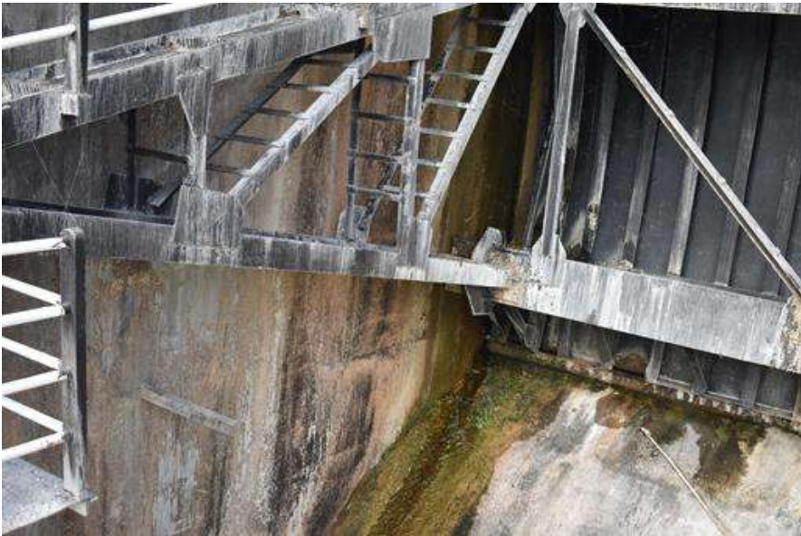
Leakage from Piers of spillway
